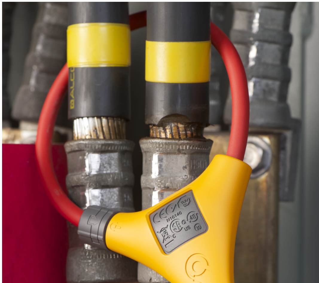
Use a flexible current probe for situations like this, where large conductors make it difficult to use the clamp meter jaws.
